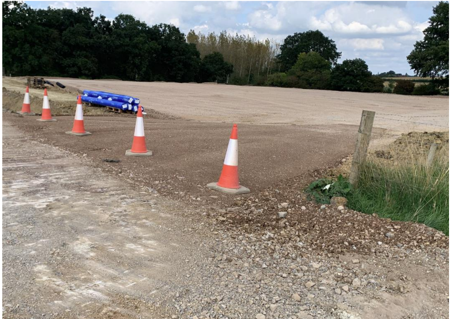
Image shows a platform which has been constructed ready for the concrete base to be poured.
